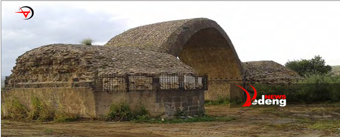
FIGURE 11. A PHOTOGRAPH OF THE BRIDGE WITH PROTECTIVE GRILLS OVER ITS DAMAGED ASTROLOGICAL PANELS, POSTED ON THE VEDENG NEWS WEBSITE ON AUGUST 27 2016.
